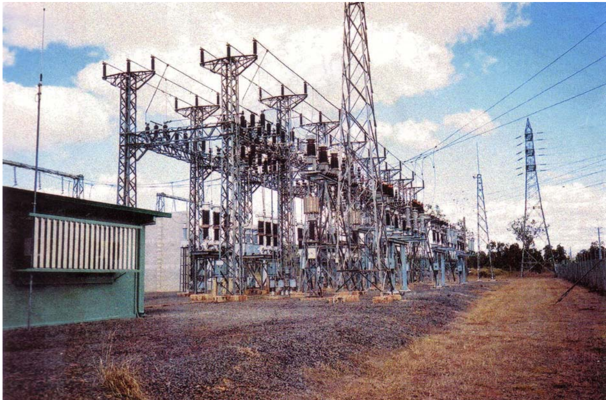
Figure 1: Turkinje Zone Substation
