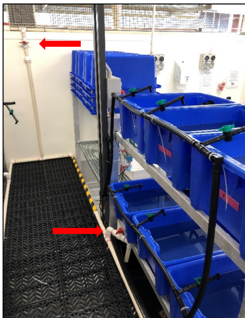
Figure 39: The Caraplace saltwater valve and a sump valve is displayed in the photo above.
