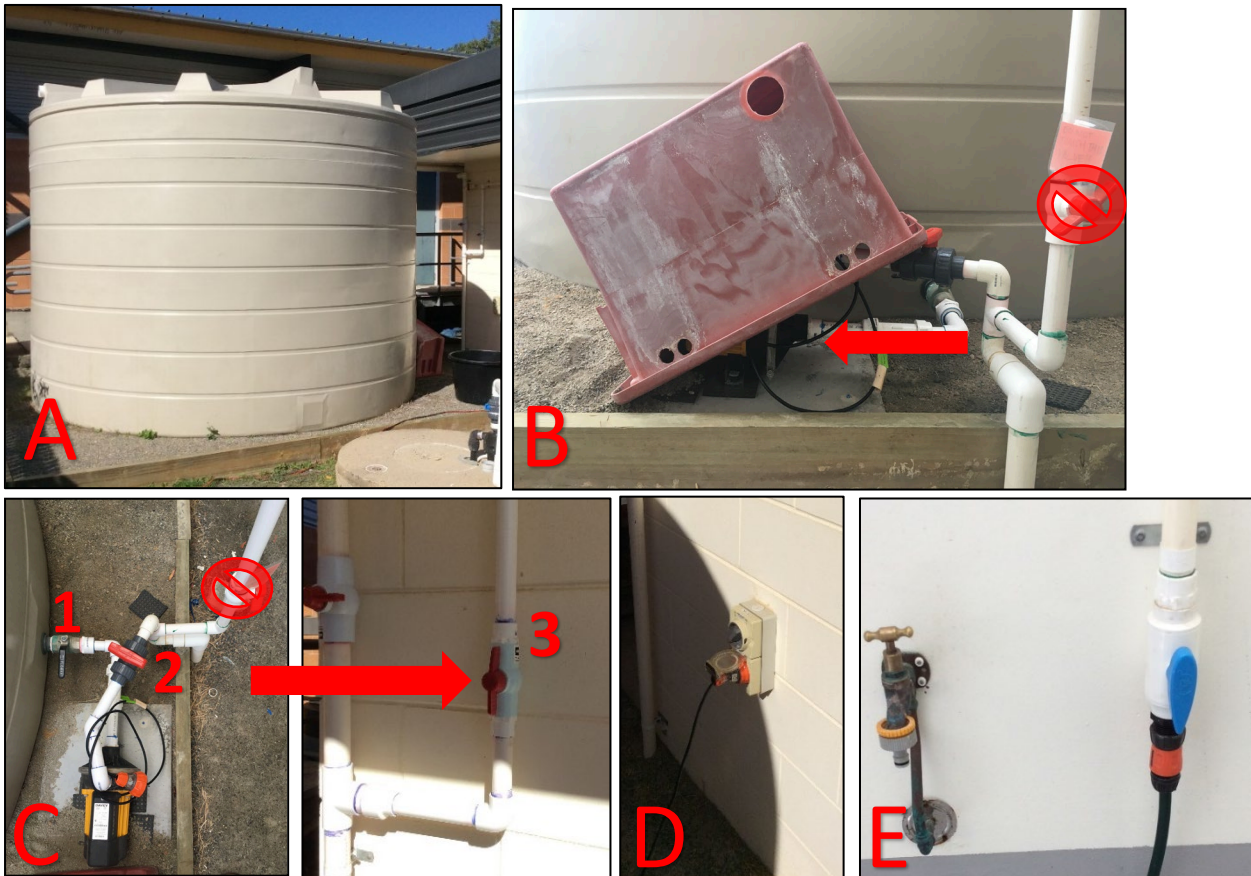
Figure 38. A) The salt water holding tank is next to building 85. You can access it by going through the gate next to the Caraplace. B) The pump is located underneath the red bin (to protect from rain and sunlight). Do not touch the valve on the PVC plumbing that acts as a pressure release valve. There is a red tag on this valve. C) Open the valve closest to the salt water tank (1), then the red valve (2), then the red valve on the building to the Caraplace (3). When the valves are open, the handles will be parallel to the plumbing. Do not touch the pressure release valve. D) Plug in the pump. E) Open the saltwater valve inside the Caraplace to flush out sitting water. Then, transfer the hose from the fresh water spout to the saltwater valve.
