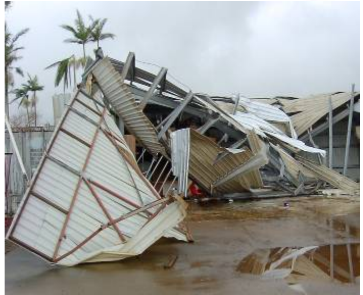
Failure of shed following Cyclone Larry
