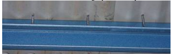
Roofing screws missed top hat batten
