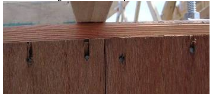
Gun nails over driven in bracing panel
