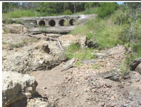
Pipe culvert in relatively steep gradient stream reach - erosion downstream (24/03/05)
