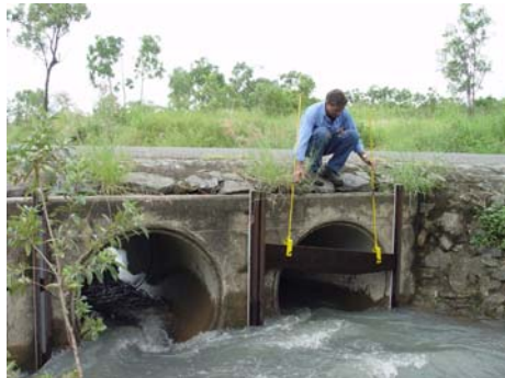
Manipulating nib wall flow control boards at culvert inlet (11/04/06)
