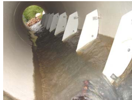
Corner “Quad” baffle fishway in Barrel 2 – looking upstream (10/04/06)
