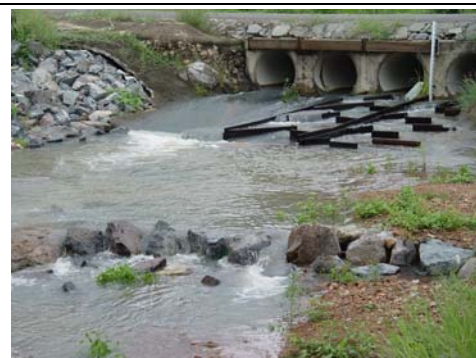
Fishway after construction – Raised tailwater level at culvert outlet due to rock ramp fishway allowing fish passage onto outlet apron (10/04/06)
