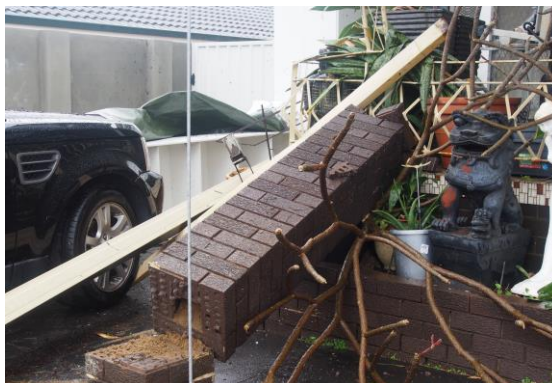
(a) Damaged carport brick pillar
