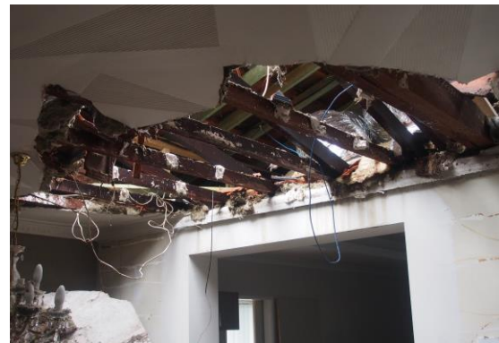
(b) Damage to ceiling
