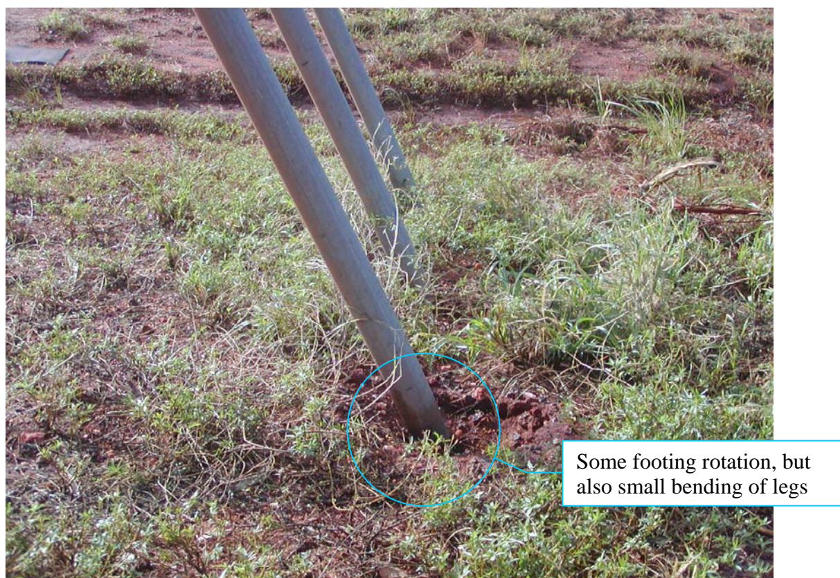
Figure 3.1: slight bend in posts of lower bound sign in Port Hedland
