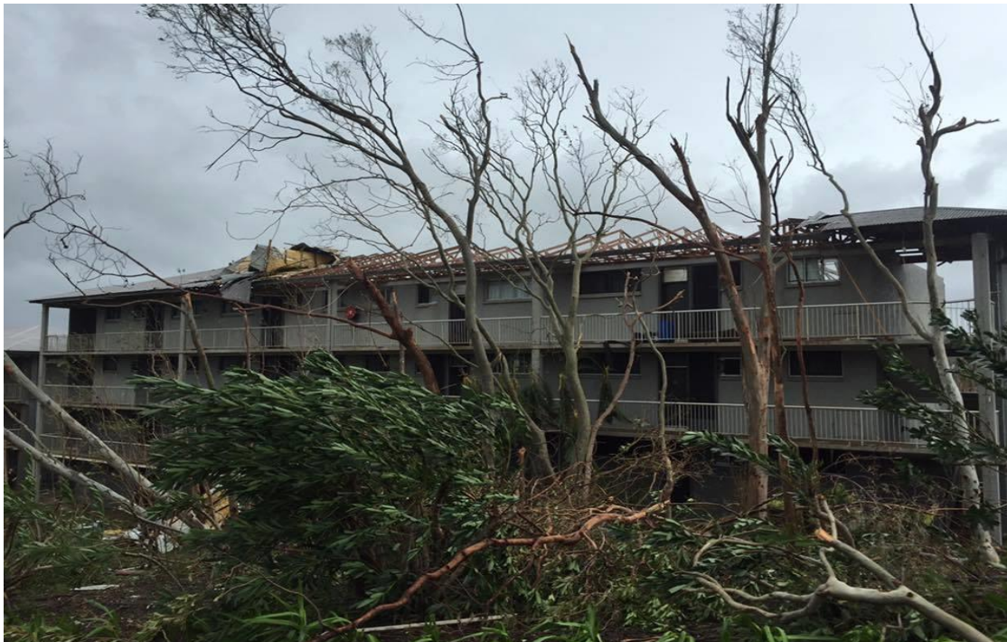
Figure 15. Loss of roof battens and cladding for a three storey unit on Hamilton Island https://www.facebook.com/7NewsBrisbane/photos/pcb.1462910670388447/1462908637055317/?type=3&theatre
