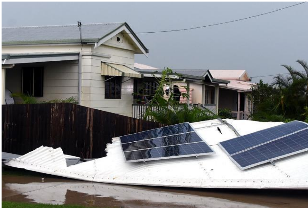
Figure 13. Large section of metal cladding (and possibly batten) failure in Bowen. Solar panel connections appear to have performed well.
