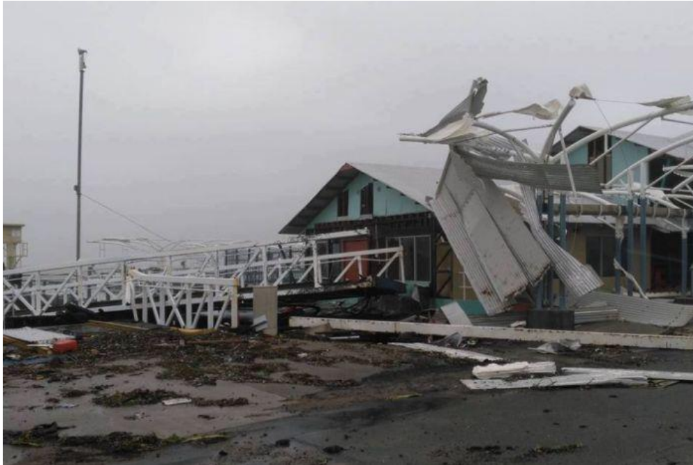
Figure 18. Failure of a canopy roof near Shute Harbour near Airlie beach
