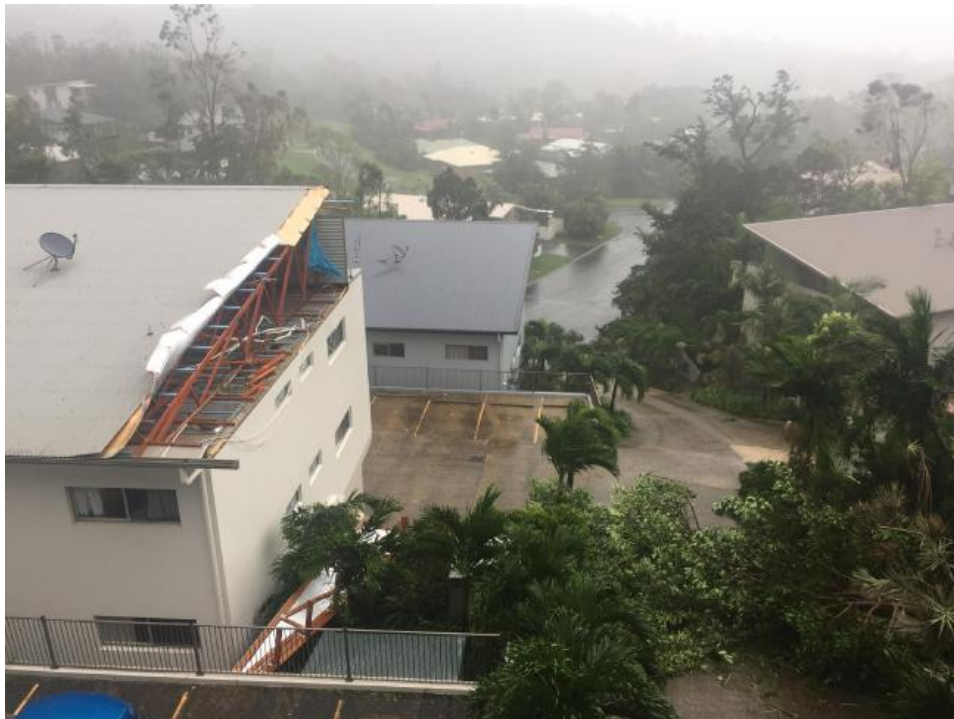
Figure 17. Failure of roof structure in the edge region for a modern apartment unit in Airlie Beach
