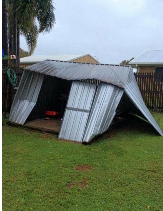
Figure 24. Damage to shed in Mackay
