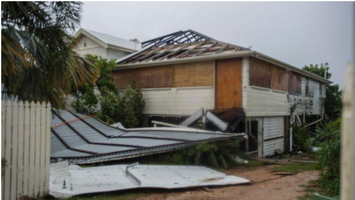
Figure 11. Structural failure of batten to rafter connections supporting metal cladding of an older high-set timber framed house (Bowen).
