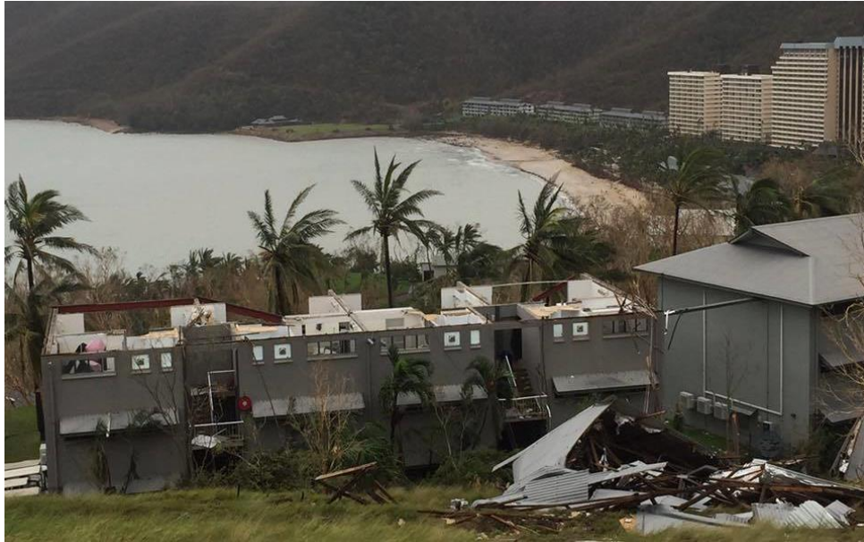
Figure 16. Complete loss of roof cladding and structure of a resort unit on Hamilton Island (likely) due to failure at roof to wall connections
