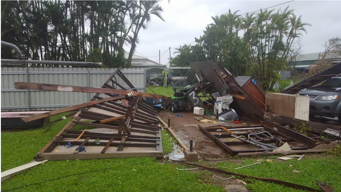
Figure 20. Failure of a timber frame carport in Airlie Beach
