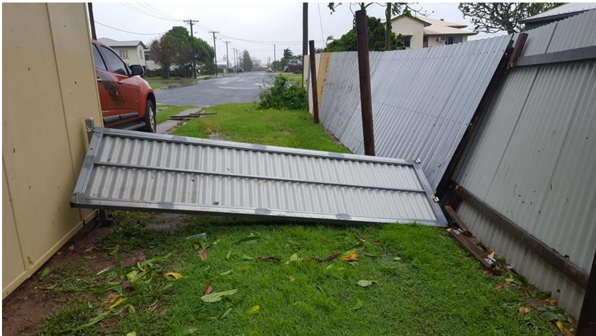
Figure 21. Damage to fencing and gates in Airlie Beach (typical)
