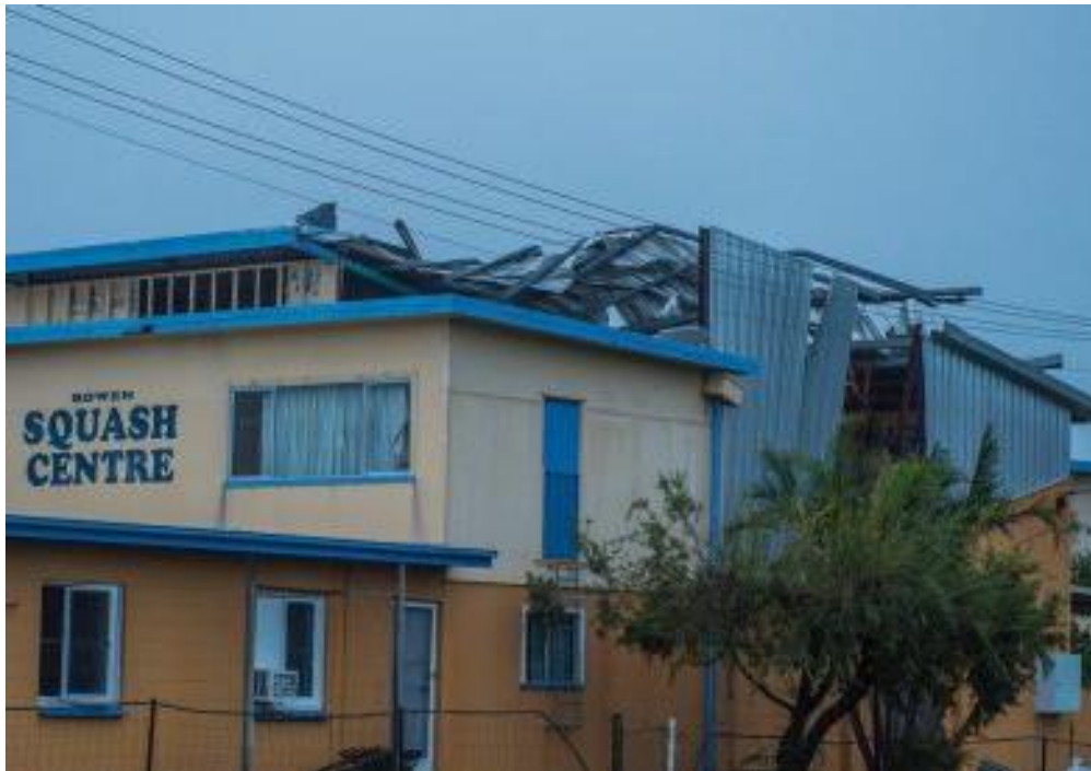
Figure 12. Failure of roof cladding and support connections due to severe wind loading (Bowen)
