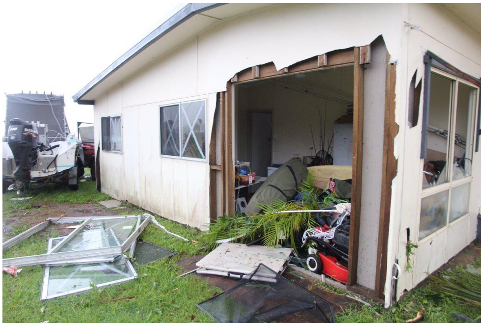
Figure 19. Failure of a large sliding door in Airlie Beach possibly due to internal pressurization following failure of the window in the windward wall (on the right in the photo)
