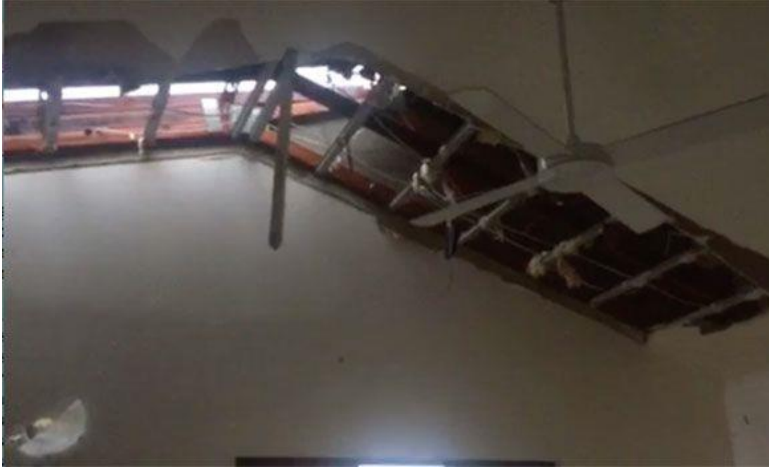
Figure 14. Damage to metal cladding resulting in water damage to a ceiling in Hamilton Island https://au.news.yahoo.com/a/34817344/cyclone-debbie-continues-to-weaken-after-unleashing-on-mainland-queensland-hitting-bowen-after-smashing-whitsundays/#page1
