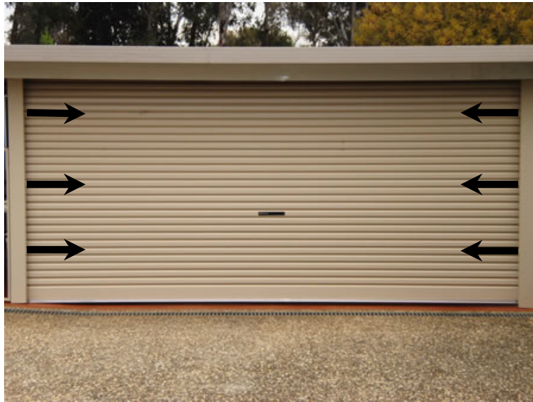
Figure 3 – The door will try to pull away from the guides as shown under wind loading. If the guides offer some form of restraint, the door may resist the wind forces by membrane action. In this case the forces in the plane of the door (shown here as black arrows) can be extremely high. These forces must be accounted for in design, or failure can occur in the guides, the fasteners or the surrounding structural frame of the building.
