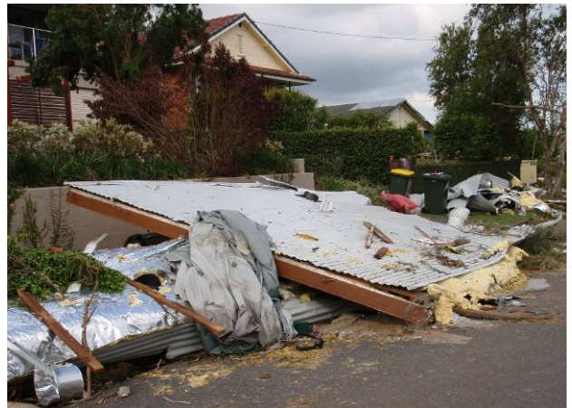
Complete roof panel lifted off house after Brisbane storms
