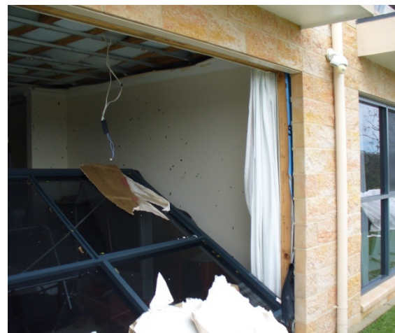
Photograph from CTS Technical Report No 55, showing window blown in as a unit as a result of poor fixing detail.
