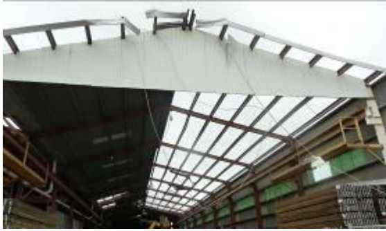
Loss of cladding, and buckled purlins
