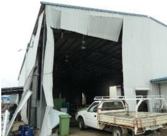
Roller door and mullion failure
