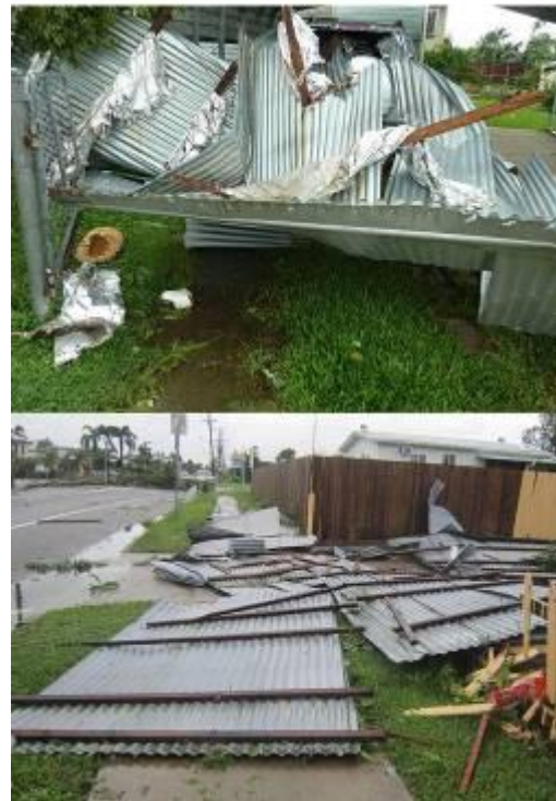
Failure of nailed batten to rafter connections
