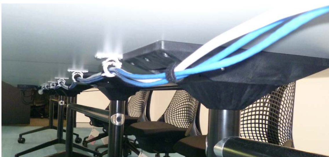
Image above showing Bar Table 1 Data and Power cable run underneath table.
