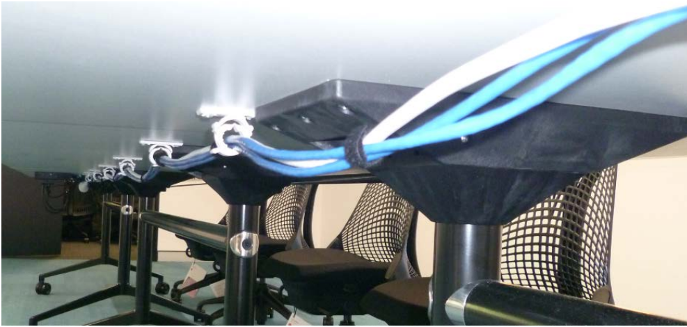
Image above showing Bar Table 1 cables run underneath tables and held in position by carrier/hooks.
