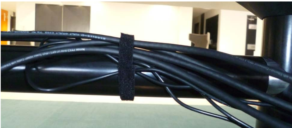
Image above showing excess cables secured using Velcro ties.
