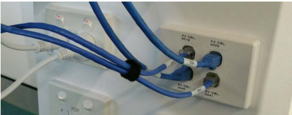
Image above showing Bar table connection to sockets on column. Data outlets 19, 20, 40 and 41 plus 2 x power.
