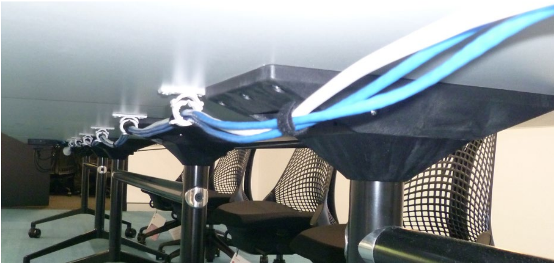
Image above showing Bar Table 1 Data and Power cable run underneath table.
