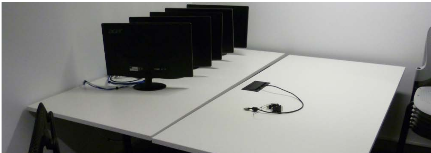
Image above showing Bar tables 1 with 5 Preview Monitors and long cable loom plus Bar table 2.
