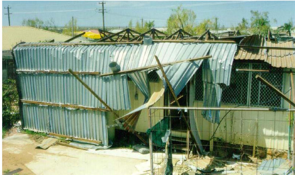
Figure 1: Roof failure following Cyclone Vance
