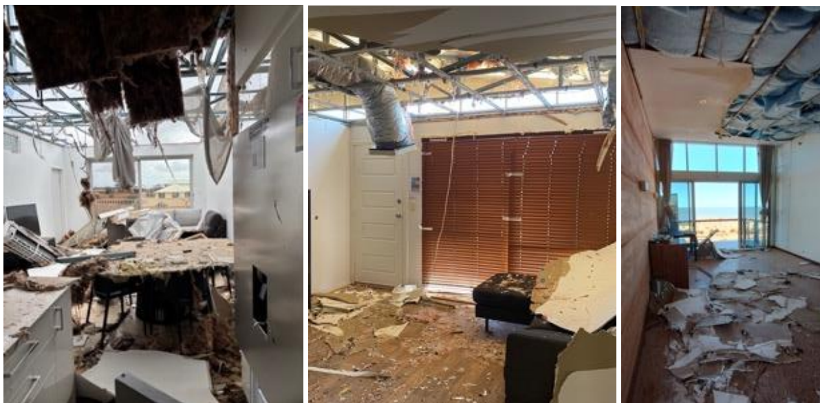
(a) Missing roof
