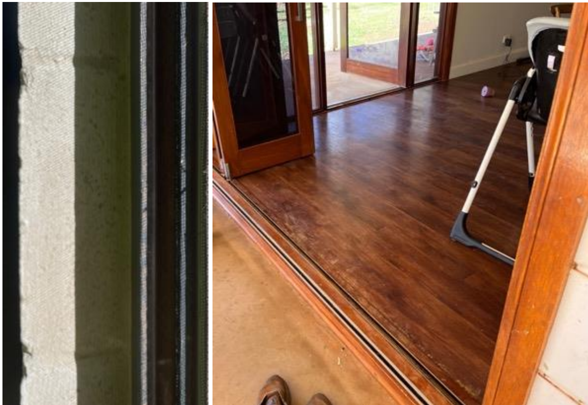
(a) Water between window and blockwork (b) Water under bifold doors
