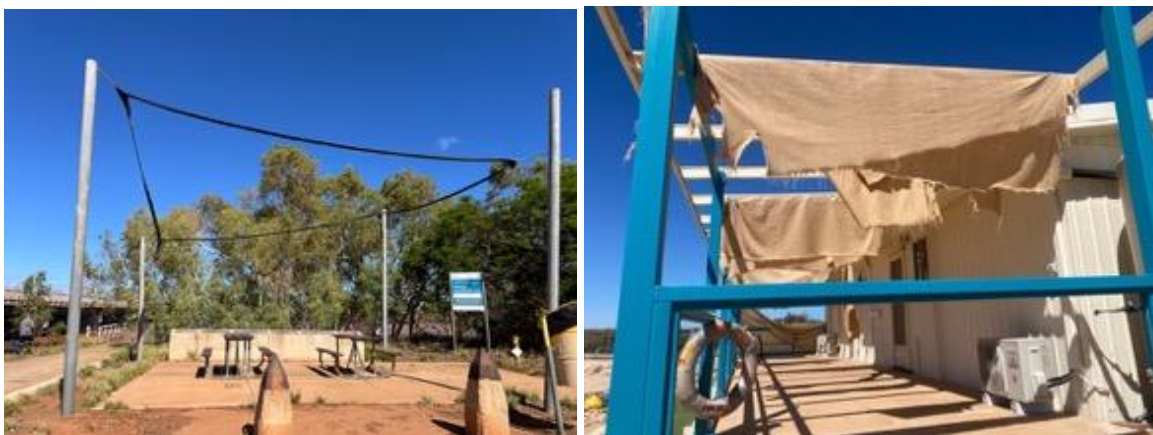
Figure 6-35 Damaged shade sails that had not been taken down in preparation for the cyclone
