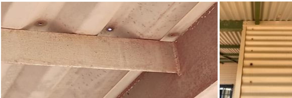
(b) Corrosion of cladding fasteners leading to fastener failure
