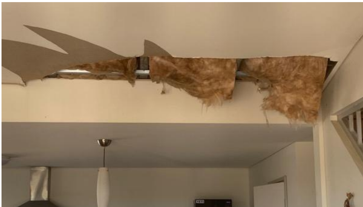
Figure 8-4 Ceiling damage under a box gutter in a house
