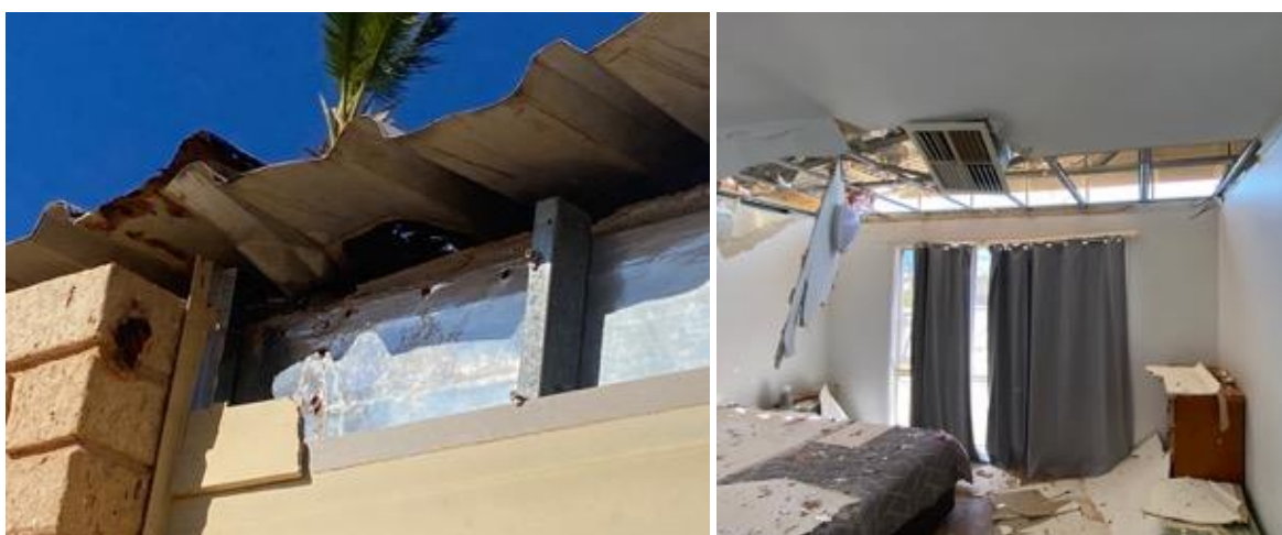
Figure 6-19 Water entry following veranda loss
