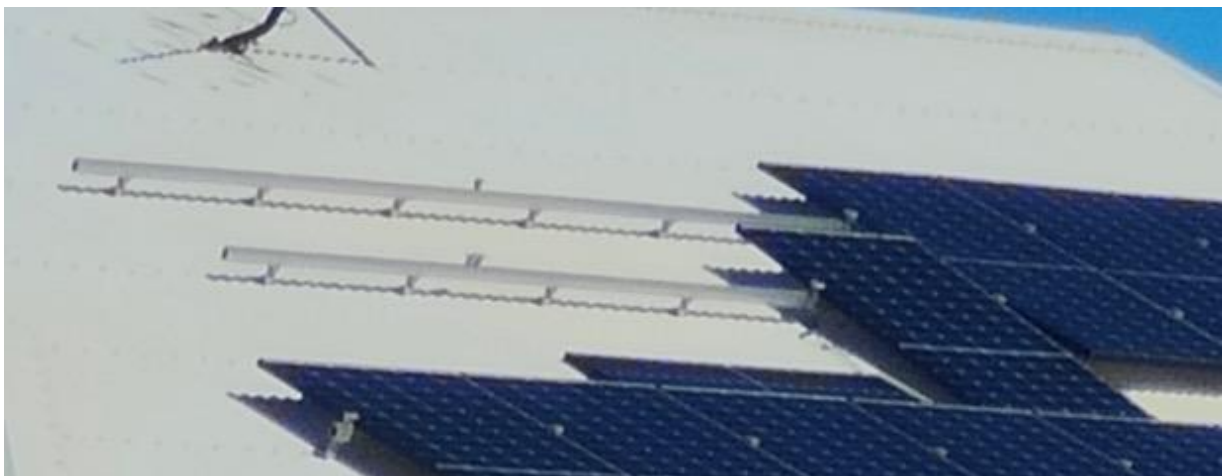
(b) Some detached panels still on the roof
