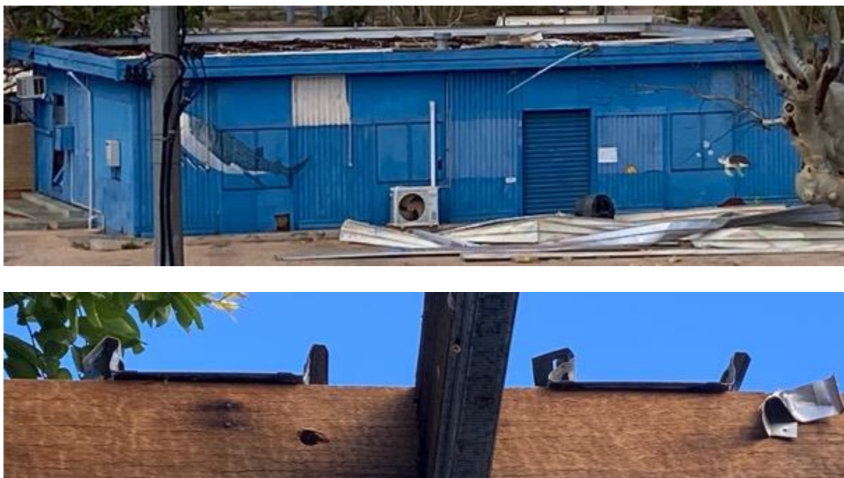
Figure 6-4 Loss of older concealed fixed roofing
