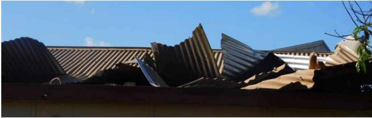
(a) Partial roof failure due to deterioration of roofing fasteners
