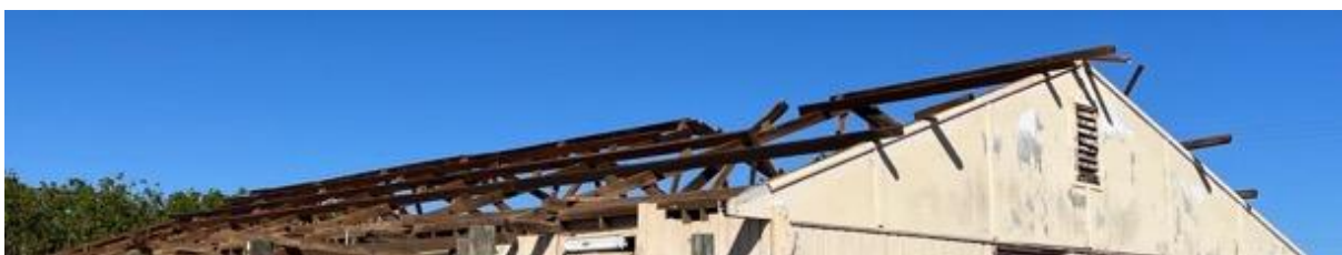
Figure 6-11 Failure of some purlin to truss connections
