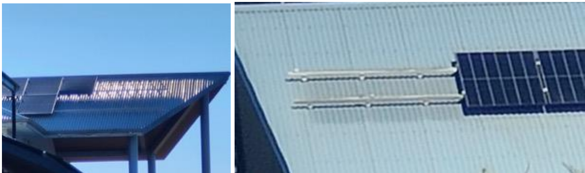
(c) Missing detached panels
