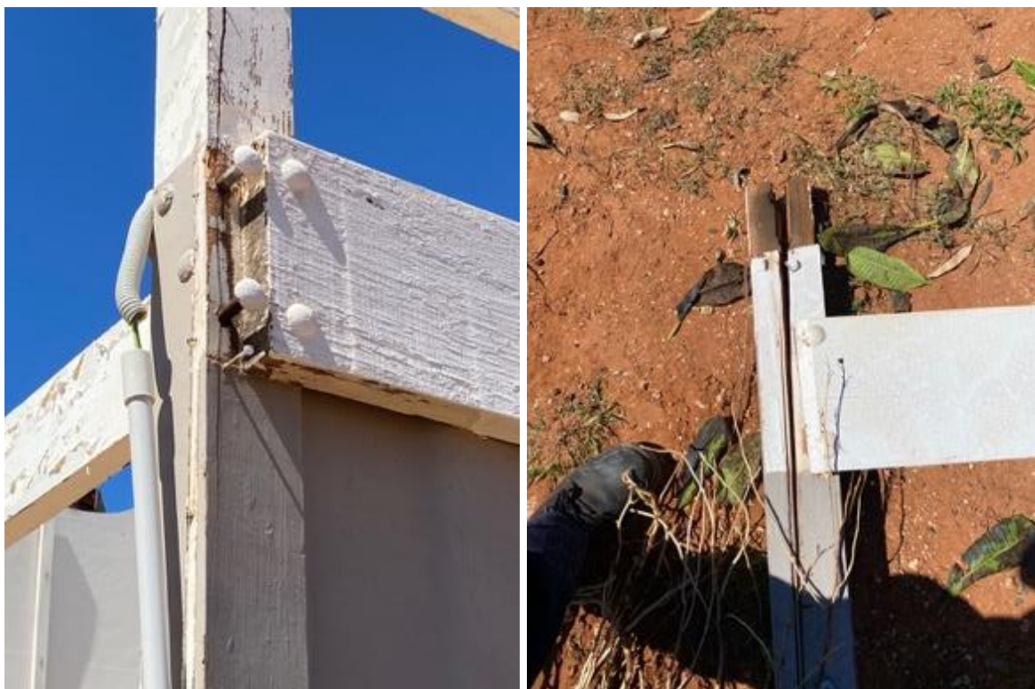
Figure 6-18 Insufficient end distance for bolts on veranda beams
