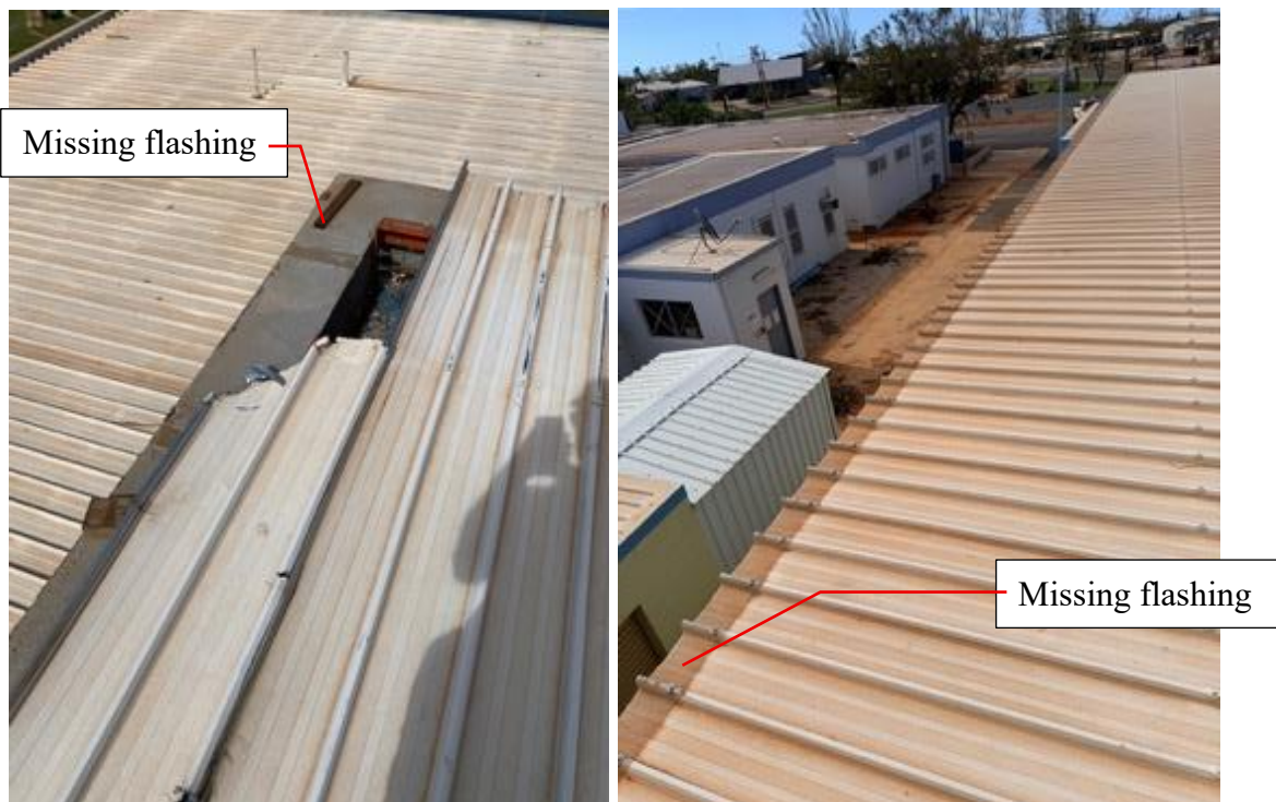
(a) Flashing parallel to ribs Figure 6-1 Missing flashings
