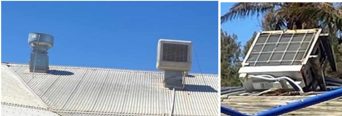
Figure 6-22 Roof-top air conditioners and kitchen extractors
