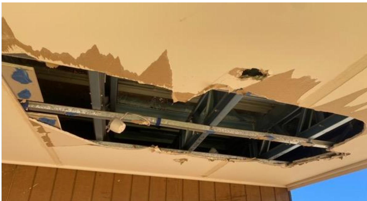
Figure 8-3 Water damage of external plasterboard ceilings
