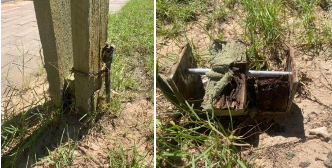
Figure 6-16 Rotten veranda posts
