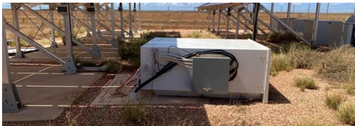
Figure 6-27 Damage to ground mounted cabinets
