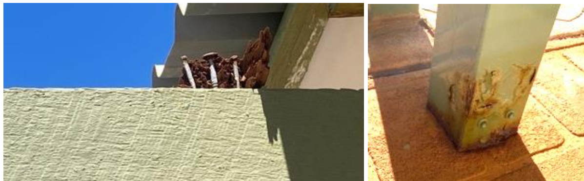
(a) Rot in batten
