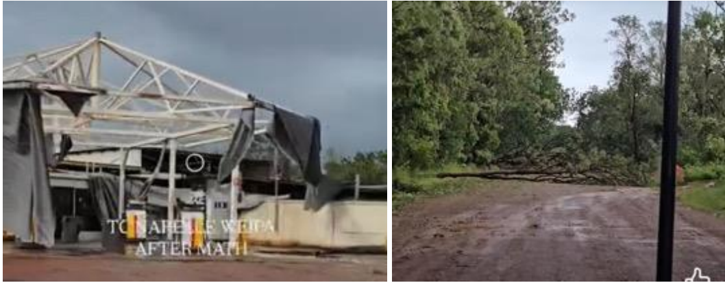
Figure 4-1 Social media images of damage from Weipa
