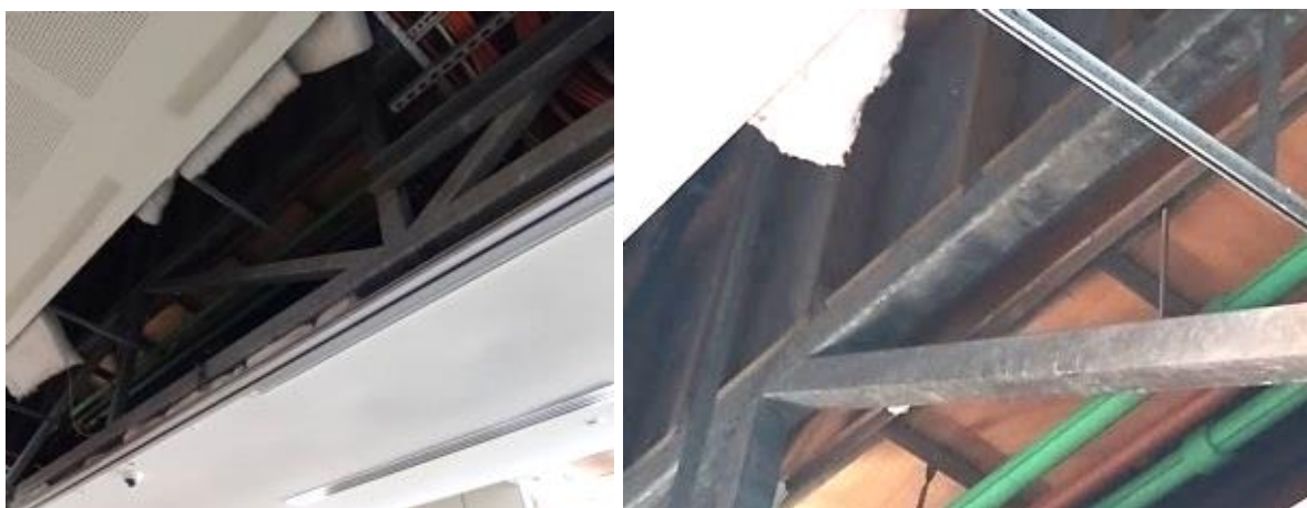
Figure 8-5 Ceiling damage under a box gutter in a commercial building
