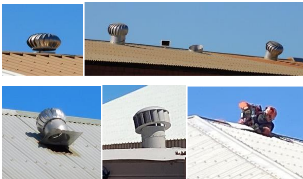
Figure 6-21 Damage to rooftop ventilators
