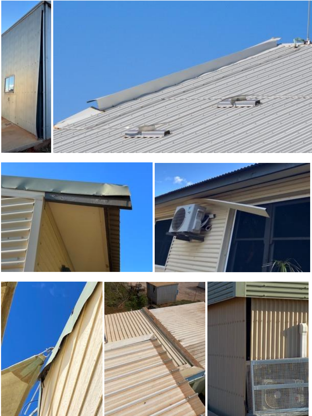
Figure 6-23 A collage of damaged flashings from TC Narelle
