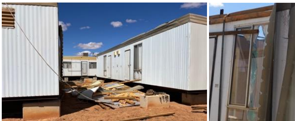
Figure 6-9 Roof loss in one donga that had damage to a windward window
