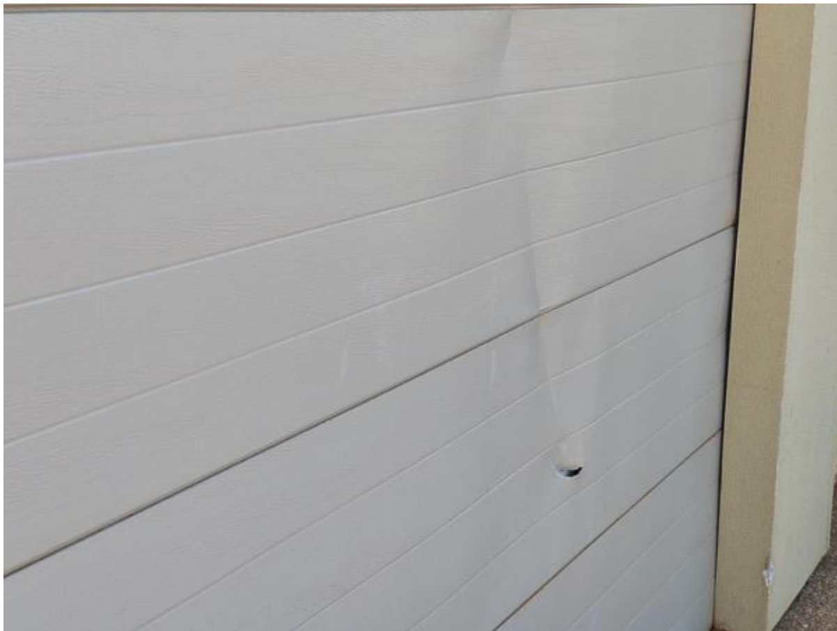
Figure 6-31 Debris damage on a garage door from an impact by a solar panel
