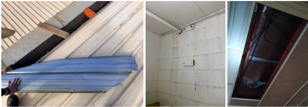
(a) Damaged roofing
