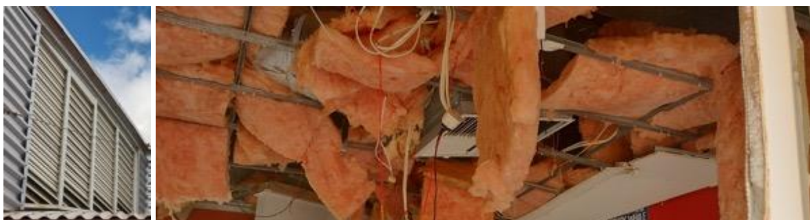
(a) Redundant vents (b) collapse of dry ceiling
