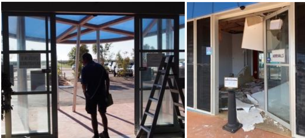
(a) In TC Olwyn Figure 8-12 Failure of automatic sliding glass doors
