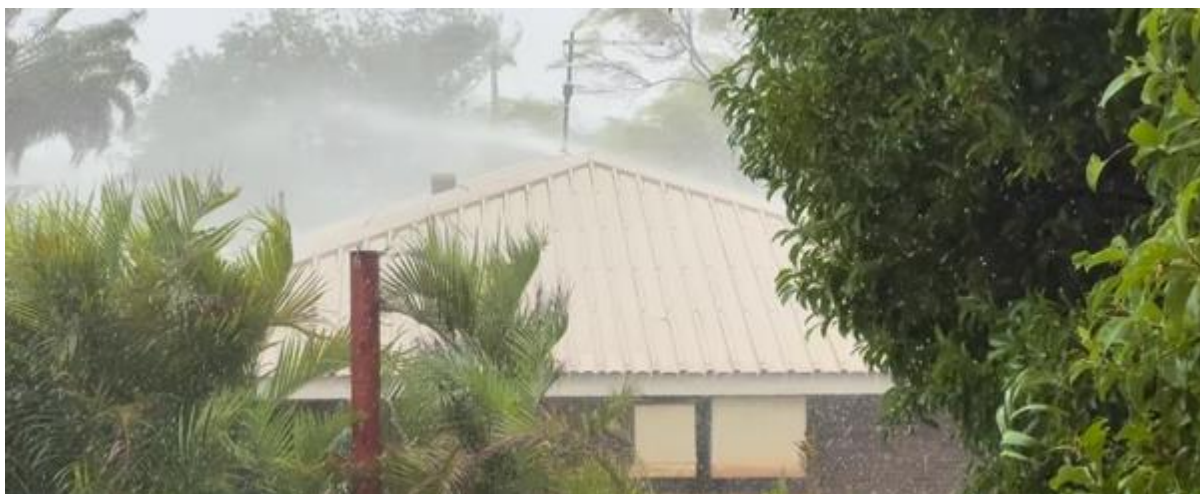
Figure 8-2 Water driven up a roof slope in TC Narelle
