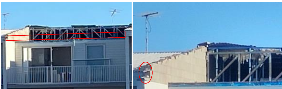
(a) Roof loss
