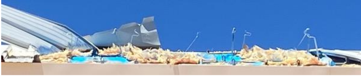
Figure 6-5 Failure of contemporary concealed fix roofing
