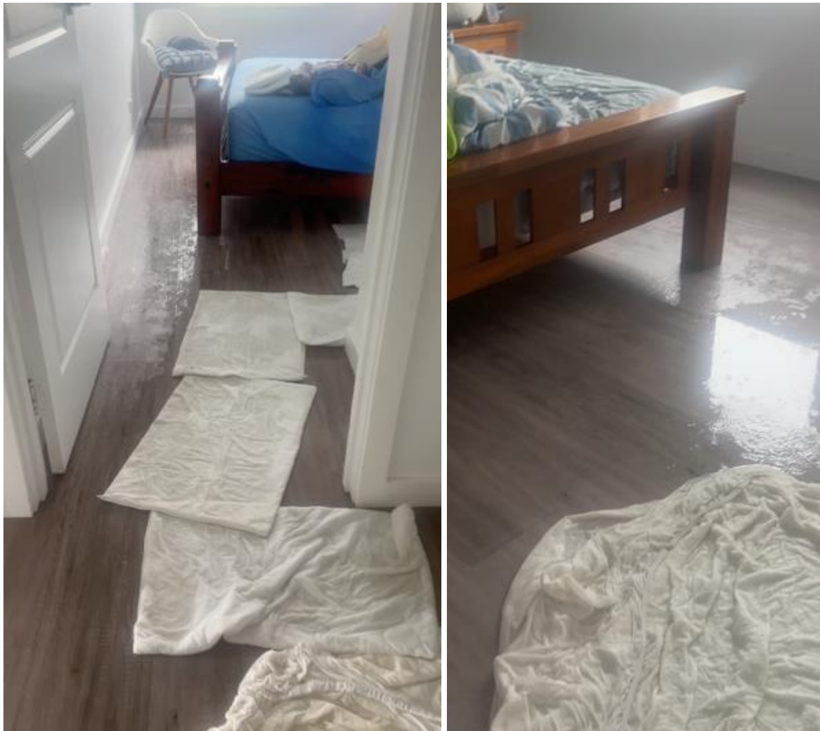
Figure 8-6 Water falling from the ceiling under valley gutters during TC Narelle
