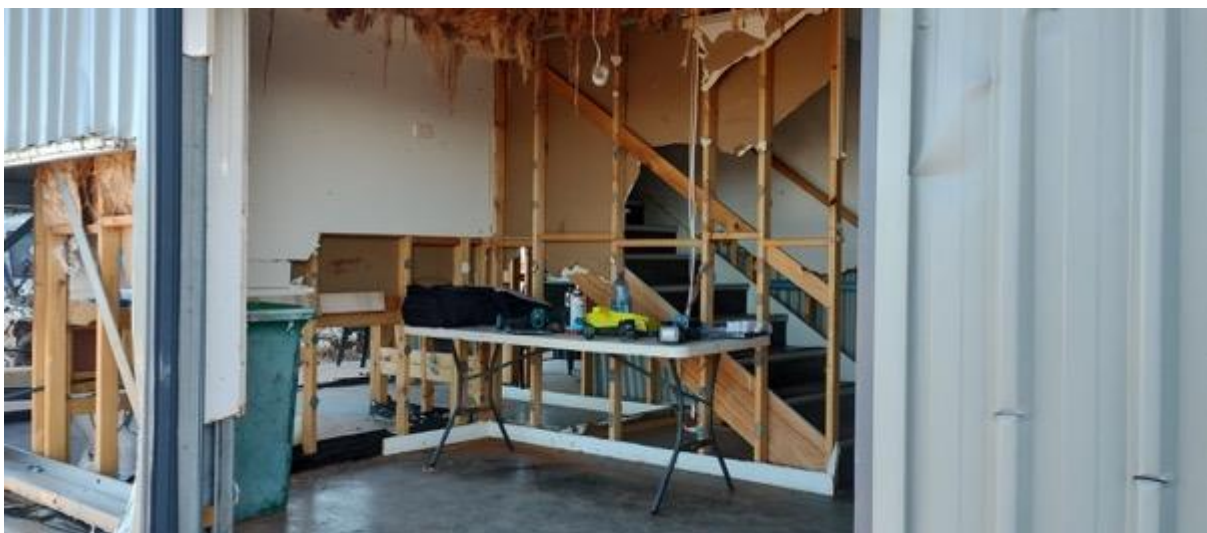
Figure 7-6 Wave damage to office warehouse, Exmouth
