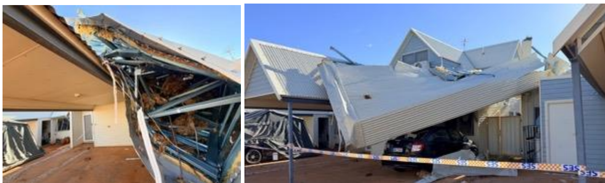
Figure 6-32 A section of roof as wind-borne debris
