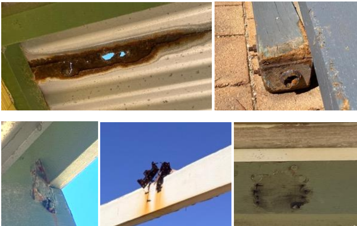
Figure 6-17 Corrosion in steel elements of verandas
