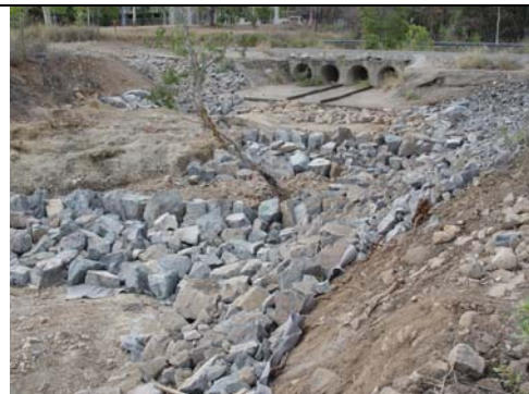
Rock ramp / cascade fishway constructed downstream of culvert to raise water levels in downstream channel – apron fishway under construction (17/12/05)
