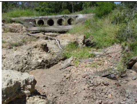
Fish migration barriers at existing structure due to water surface drop and high velocity shallow flow at culvert outlet apron (24/03/05)
