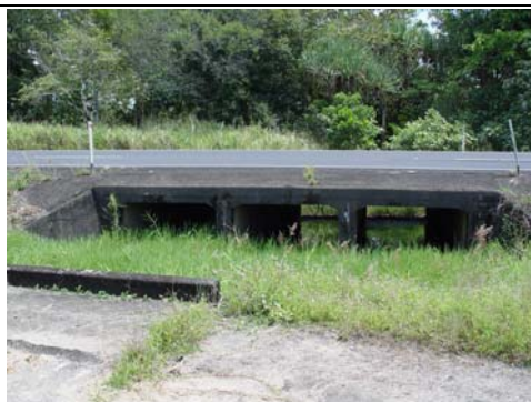
Box culvert crossing of existing Bruce Highway at waterway / fish movement corridor south of Lagoon Ck (29/09/05)
