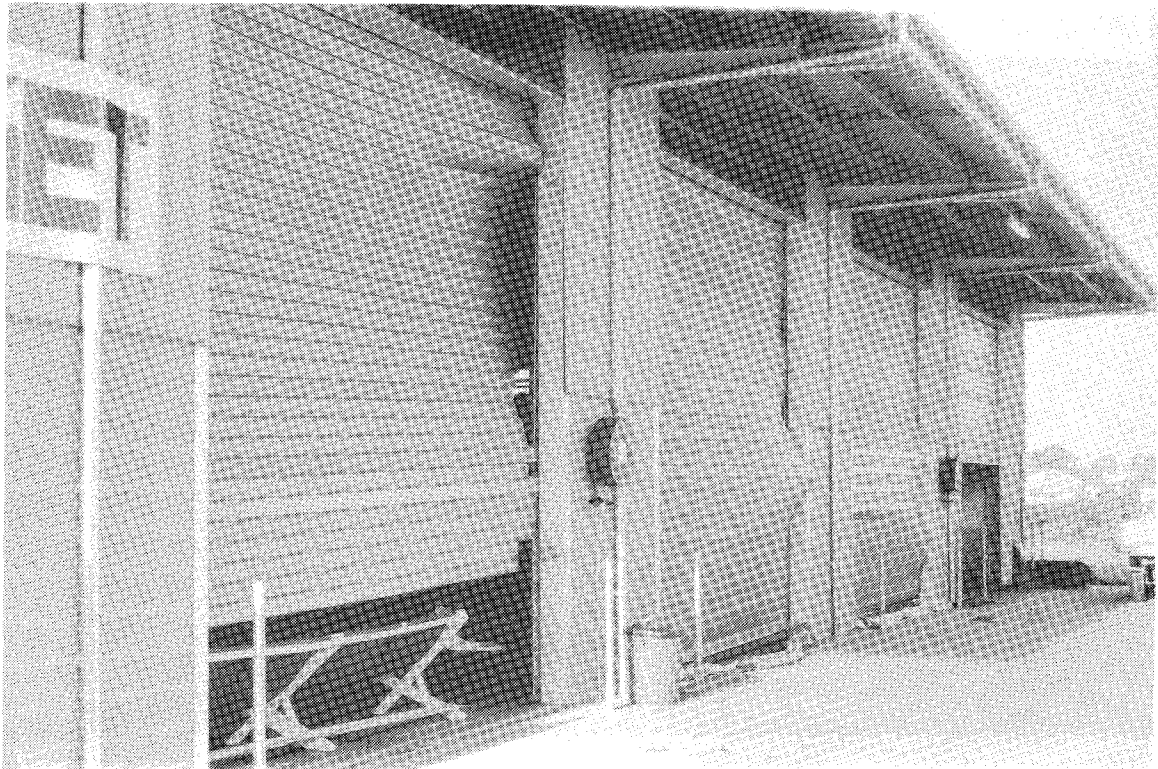
Figure 16. Damaged Roll-away Doors
