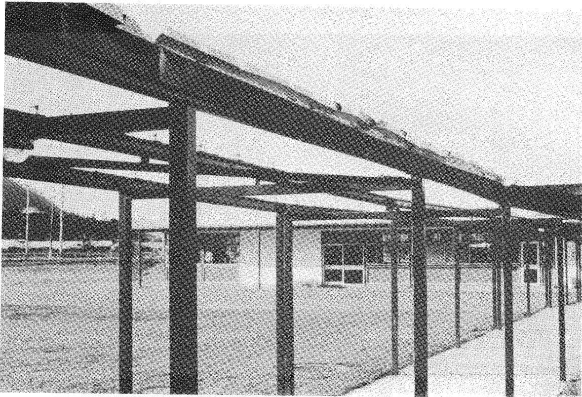
Figure 18. Secret Fixed Roofing Blown Off Walkway
