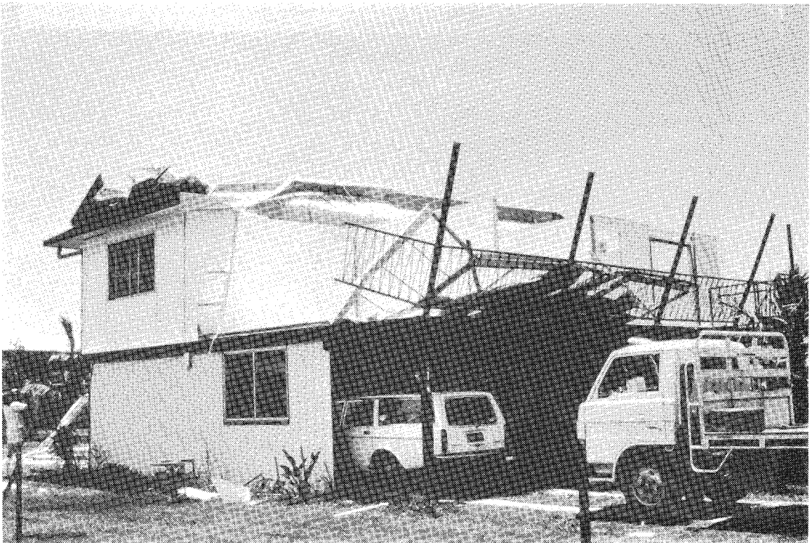
Figure 14. Damage to Panelized House
