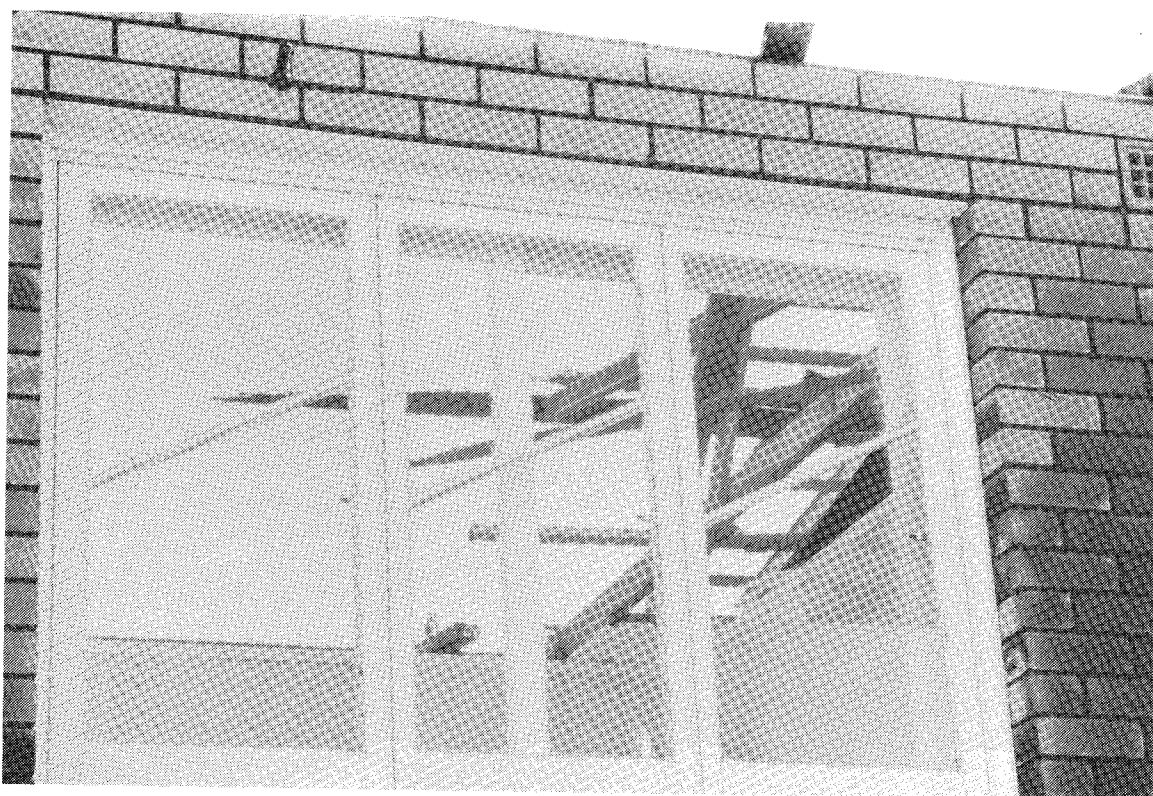
Figure 26. Roof Damage to Flats, Innisfail
